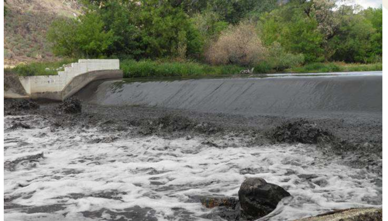
2013 High Park Fire Impacts at Greeley's Poudre Diversion
